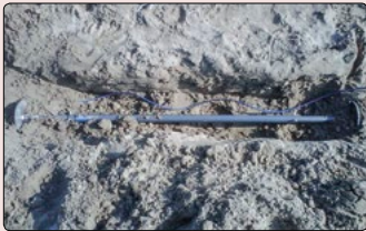
• Model 4430 Vibrating Wire Deformation Meter installation.
